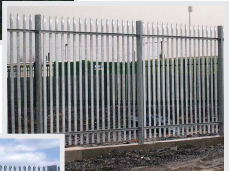
Close up of the NRA spec palisade fence panels mounted to an ST2 grade concrete plinth.
