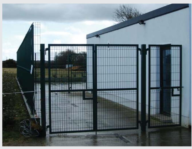
Double leaf gates and a single gate installed side by side.
